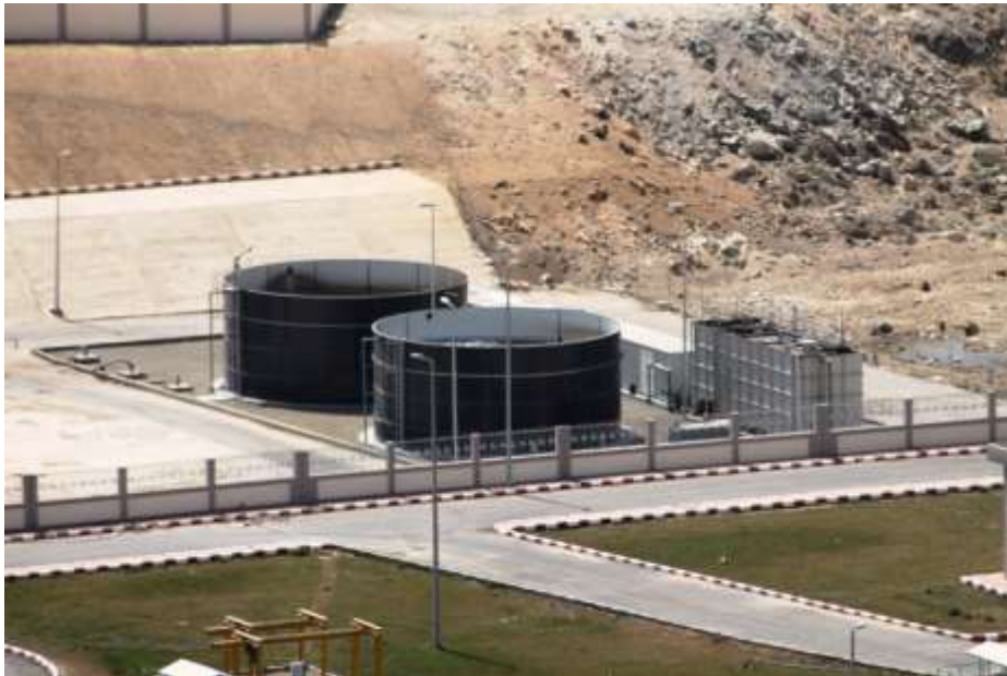
Baha MBR Package Plant.
